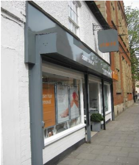
Left: A poorly designed security shutter which has a 'tacked on' appearance and adds an unsightly bulky addition to the shop frontage. This will also deaden the frontage when down.
