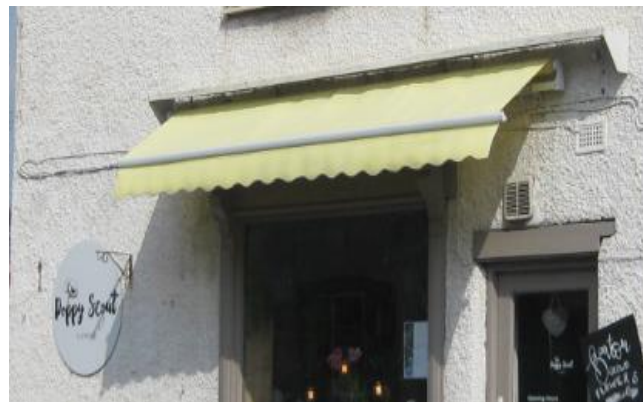
Right: Example of poorly designed canopy
