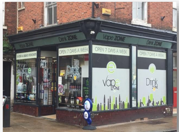
Above: While the elements of the shopfront reflect traditional design the use of extensive signage and vinyls detract from this and deaden the frontage which erodes its character.
